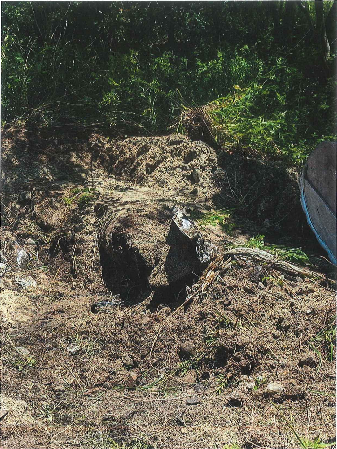
Photo 17: Large Debris below vegetative cover at TP23-10
